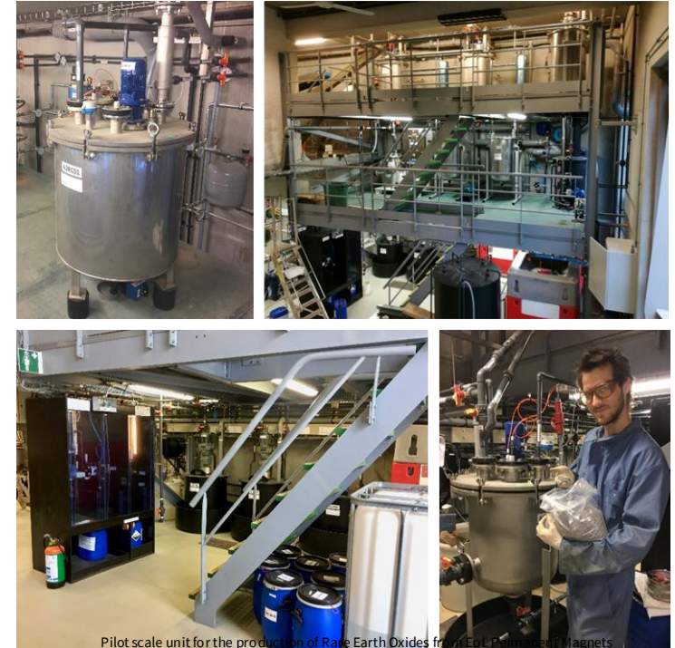
Pilot scale unit for the production of Rare Earth Oxides from EoL Permanent Magnets
